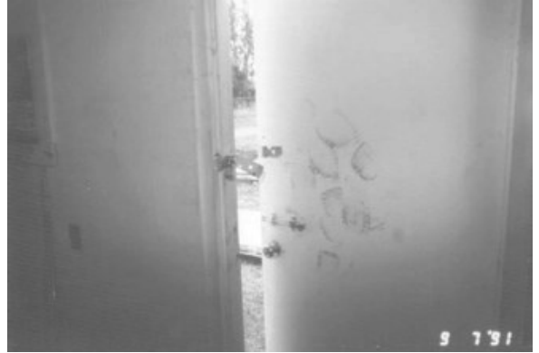
Kick marks on one of the locked doors that workers were ultimately able to escape from
